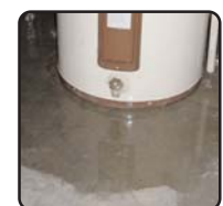
Flood Water Sensors
